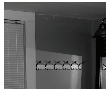
Possible Golden-rod at intersection of wall and ceiling. Governor's Mansion Leadville Colorado, Aug 09
